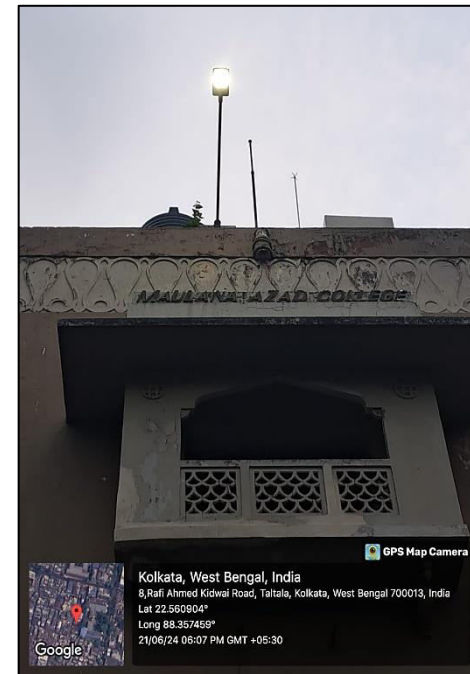
Timer controlled compound lights
