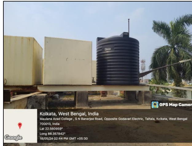
Overhead water tanks in college rooftop
