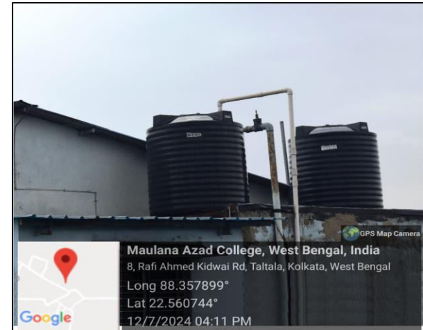
Overhead water tanks in college rooftop
