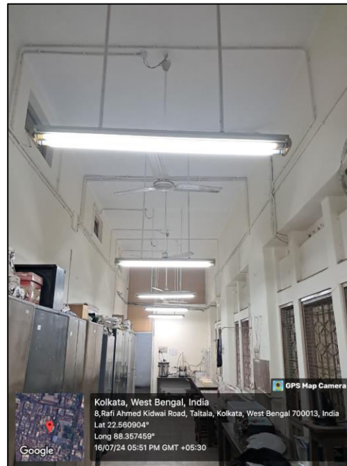
LED tube lights in corridor
