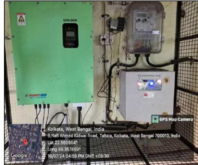
WHEELING TO THE GRID
