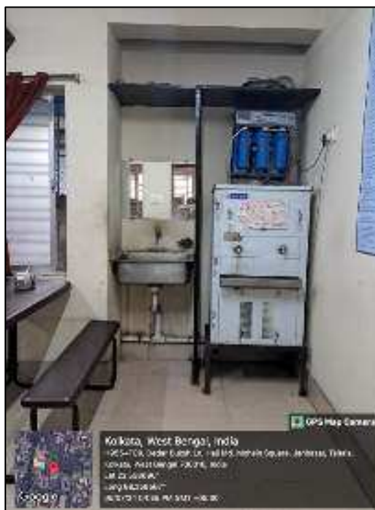
DRINKING WATER-CUM-COOLER FACILITIES
