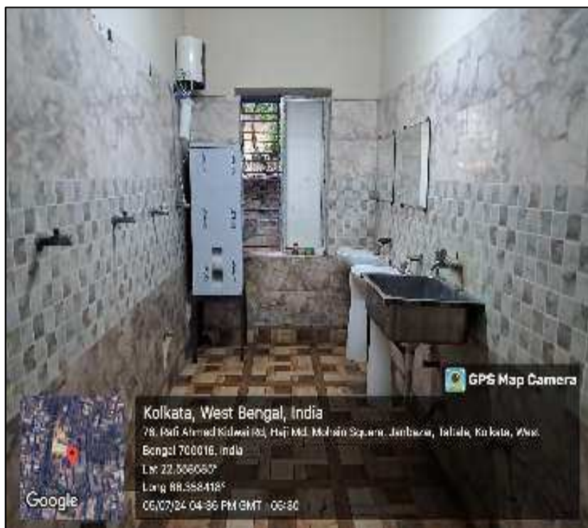
WELL MAINTAINED WASH BASINS
