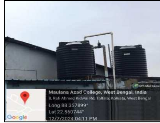
OVERHEAD WATER TANKS IN COLLEGE ROOFTOP
