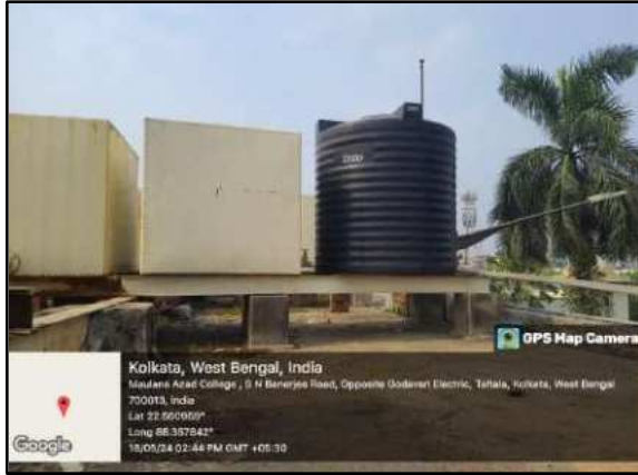
OVERHEAD WATER TANKS IN COLLEGE ROOFTOP
