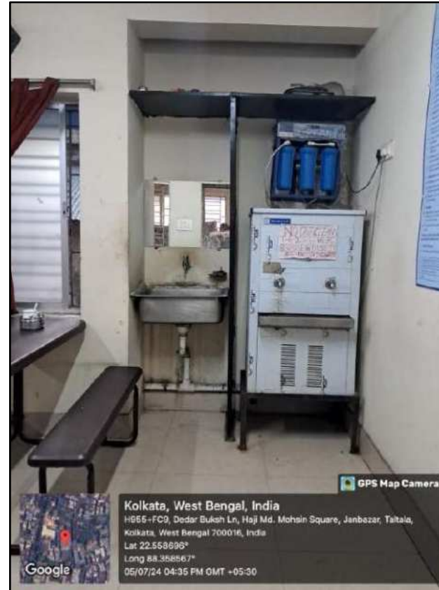
DRINKING WATER-CUM-COOLER FACILITIES
