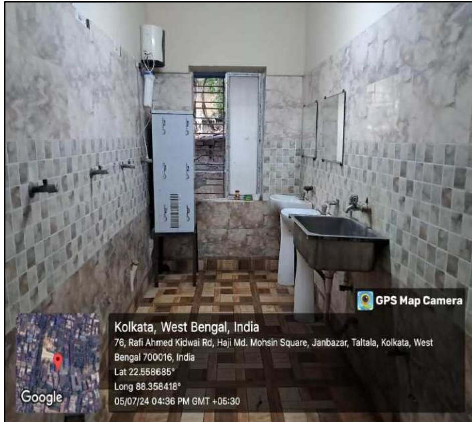
WELL MAINTAINED WASH BASINS
